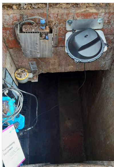
IN-CHAMBER DATA LOGGER · UK WATER UTILITY
