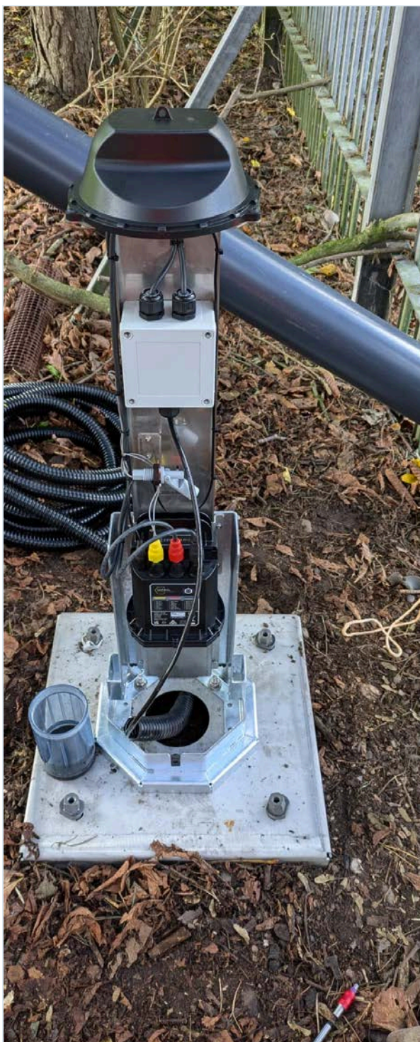
REMOTE TELEMETRY MAST · UK WATER UTILITY
