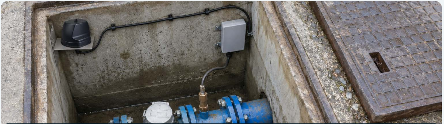
THE INSTALLED CHAMBER IS PART OF THE RF SYSTEM.
