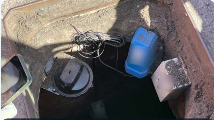
BELOW-GROUND CHAMBERS & BOUNDARY BOXES
