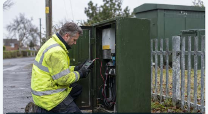
REMOTE TELEMETRY & ABOVE-GROUND ASSETS
